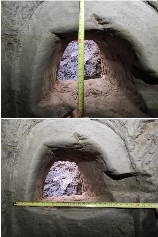
Figure 7. Measurement of the horizontal crawlway using the conventional measuring method (roll meter) (width: 43.6 cm, height: 34.5 cm) and the door frame (width: 60.7 cm).
