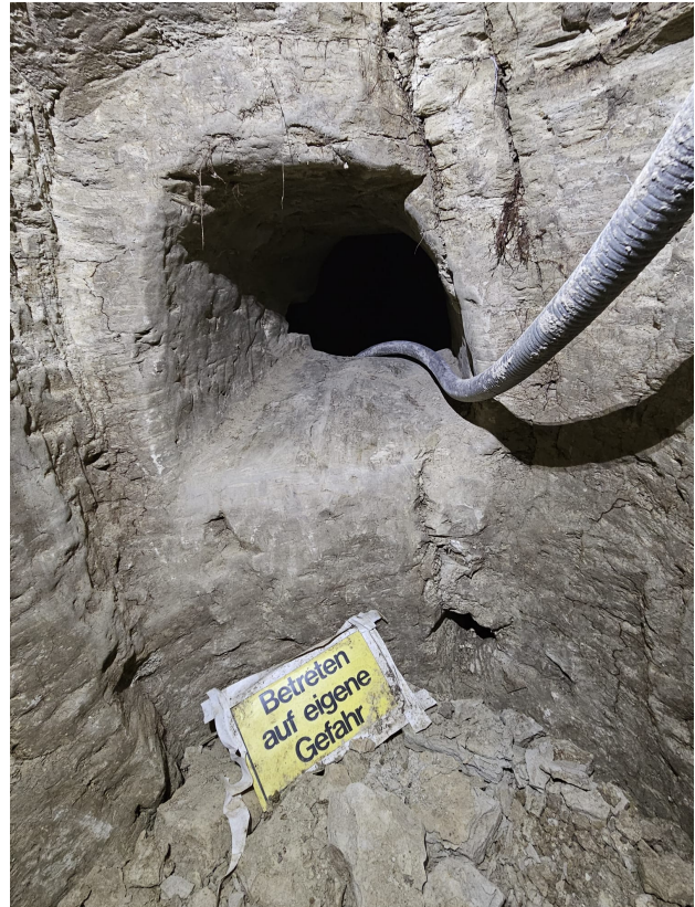
Figure 1. Confined spaces and connecting holes characterize such facilities. Due to the lack of an air shaft, a suction system would be used to supply the rooms with fresh air in order to carry out the inspection and measurement of the facility.
