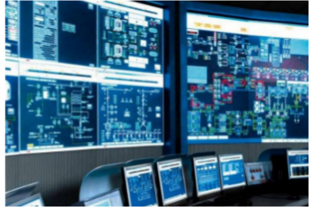
Figure 3. Example of a HMI [44]
