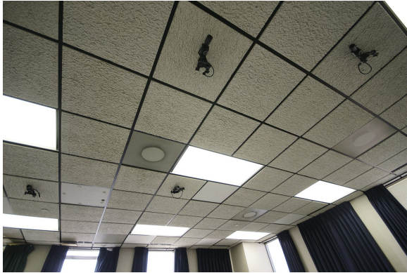
Figure 5. Some of the ceiling-mounted cameras in AVA
