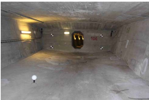
Figure 8: Sight in direction to the support 106 from the middle of the hollow box girder. On the base plate is a reference sphere and on the bulkhead of the support 106 are besides to the transition square reference points.
