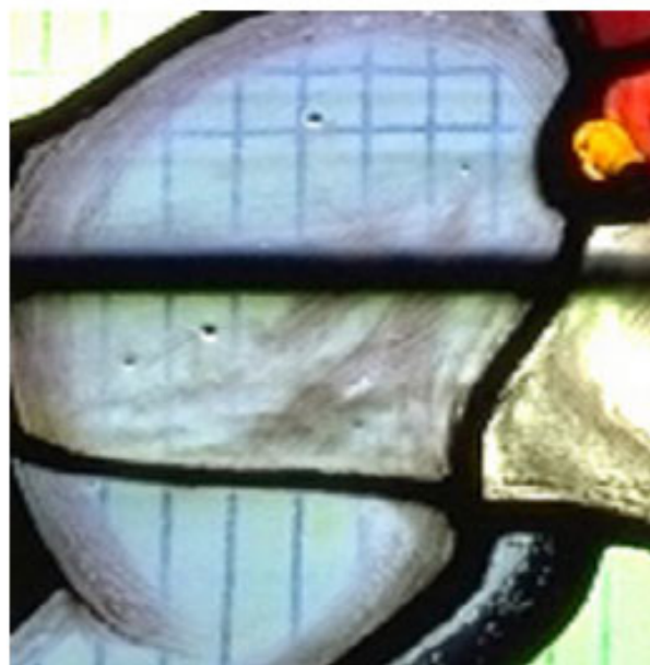
Figure 1. Shadows of horizontal support bar and wire mesh grille in a stained glass window. The detail (below) shows both the transmitted image of the grille its shadow cast by the sunlight. The window is in the chancel of the Church of St. Mary, Studley Royal, Yorkshire, UK.
