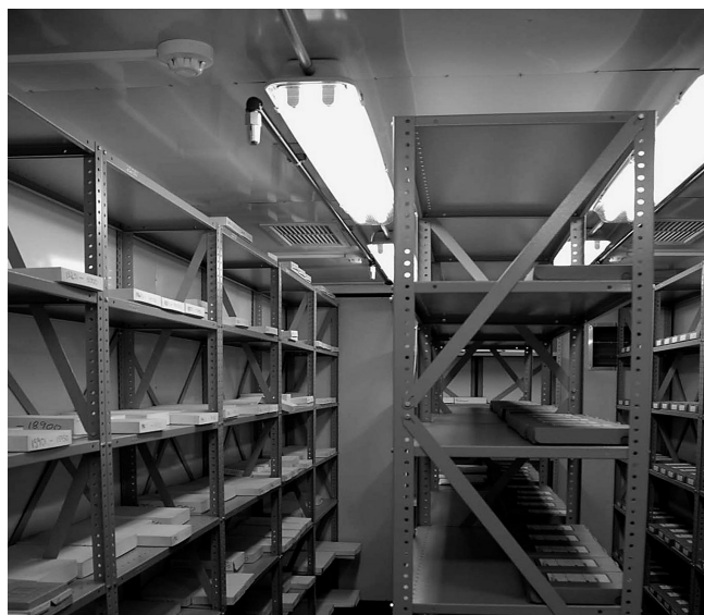
Figure 2. Nitrate film storage container of the Duggan-Cronin collection, Kimberley, showing the fire warning and CO 2 extinguishing system.
