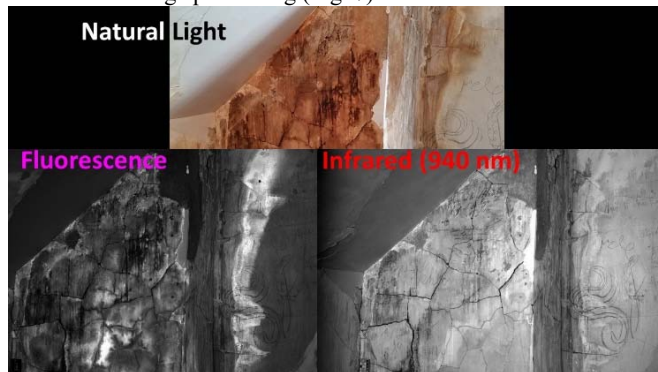
Figure 7. Captured images of a water-damaged attic ROI in Historic Blenheim in natural light, short wavelengths with filters, and infrared 940nm light
