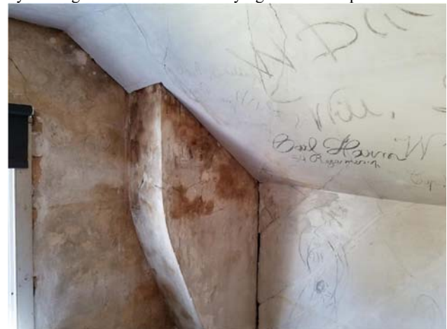
Figure 1. Attic area of Historic Blenheim with graffiti by Union Soldiers from the Civil War and environmental damage to the walls and chimneys.
